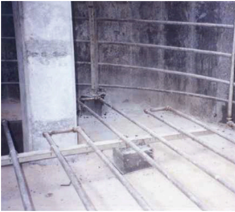
1. Steam pipes that are used to dissolve the sulfur when the sulfur pit is in full operation.
