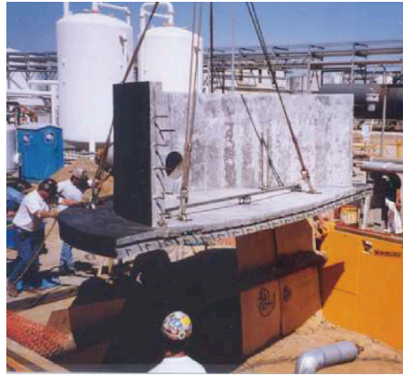
2. Installation of the first half of the sulfur pit being lowered into the ground.
